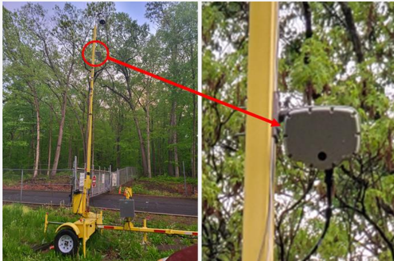
Mobile Trailer with traffic microwave sensor
