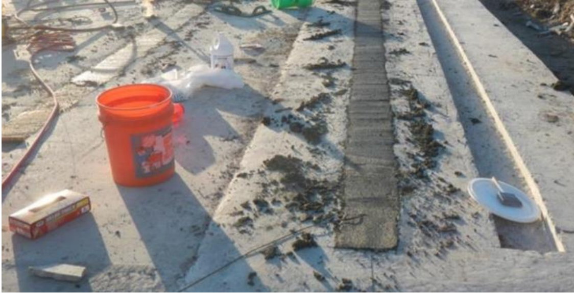
Figure 8. Field test slab with long rectangular defects being repaired similar to partial depth (13)
