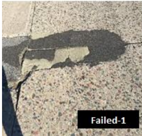
Figure 7. Photos showing condition ratings (adapted from (7) )
