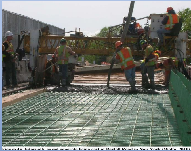
Figure 45. Internally cured concrete being cast at Bartell Road in New York (Wolfe, 2010).
