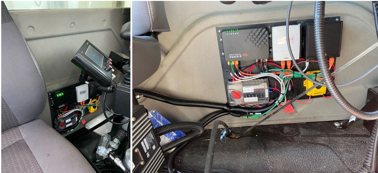
Figure 13. The camera main unit (Axis F41), PoE injector, cellular LTE modem, and the power distribution unit installed against the back wall of the cab interior in a plow dump truck (Source: NJIT)
