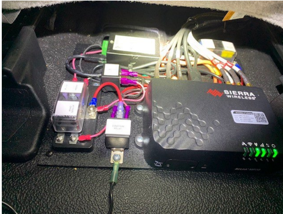
Figure 16. The electronics board without the video processing unit (not required for the dome camera models), installed under the passenger seat in F350 SSP vehicle (Source: NJIT)
