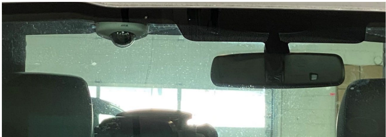
Figure 17. Dome camera (Axis P39 Series) installed in an NJDOT fleet pick-up truck – front view (Source: NJIT)
