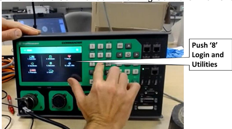
Figure 4. Trafficware Commander Initializing Controller-Utilities
