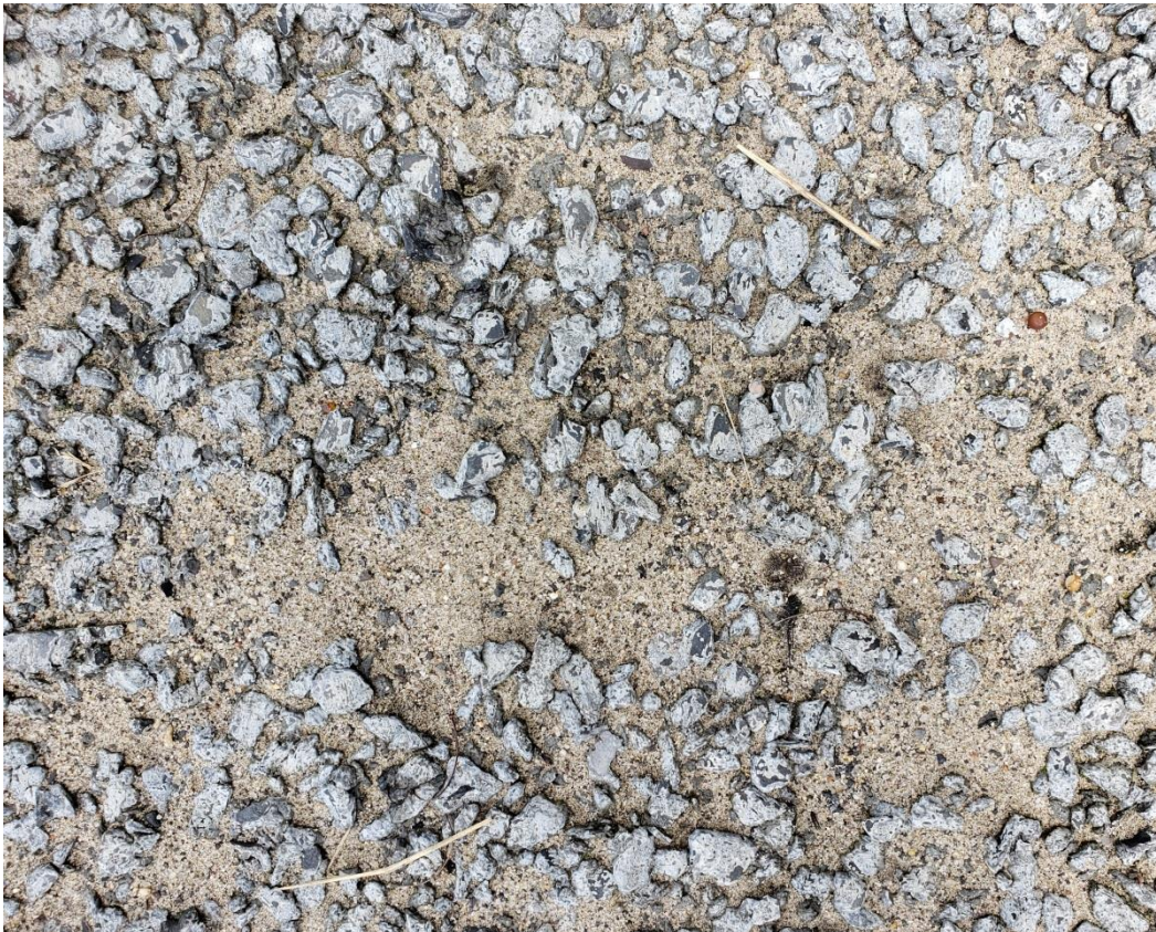
Figure 7. Severe clogging and severe raveling (Location C)
