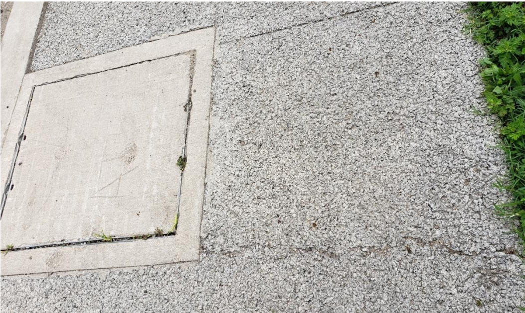
Figure 5. Porous concrete surface showing a crack initiating from the corner of the utility manhole (Location B)
