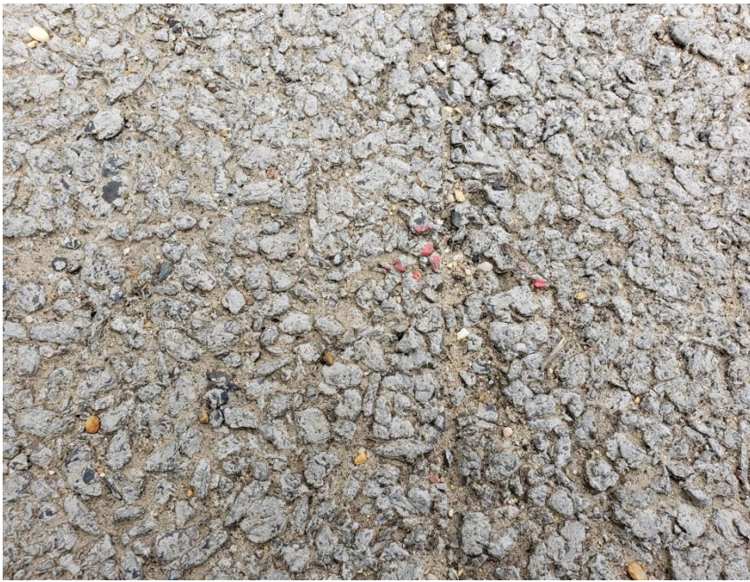
Figure 6. Medium to severe raveling and clogging (Location C)
