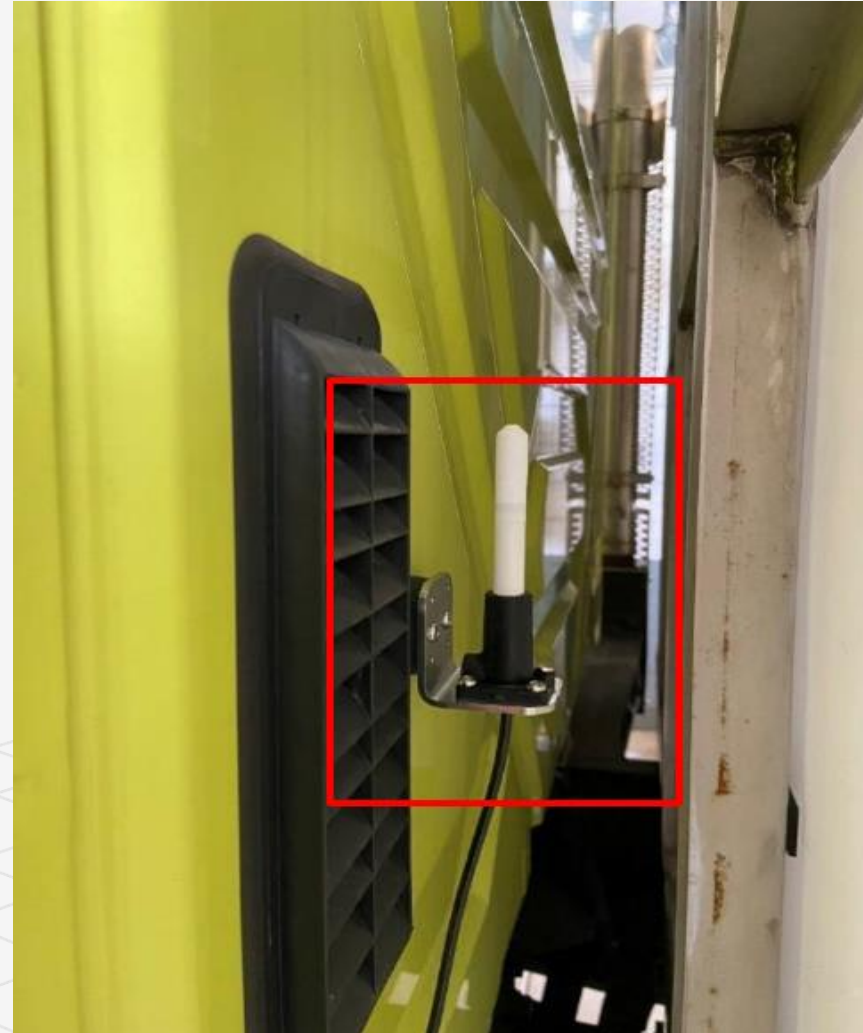
Ambient Weather Sensor Installed
